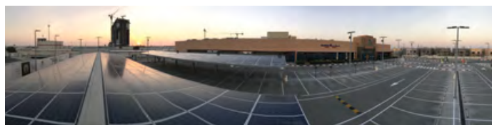
Enerwhere solar installations at MyCityCentre Al Barsha
